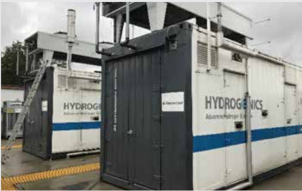
Kitty Brewster Hydrogen Production Station – Aberdeen City
