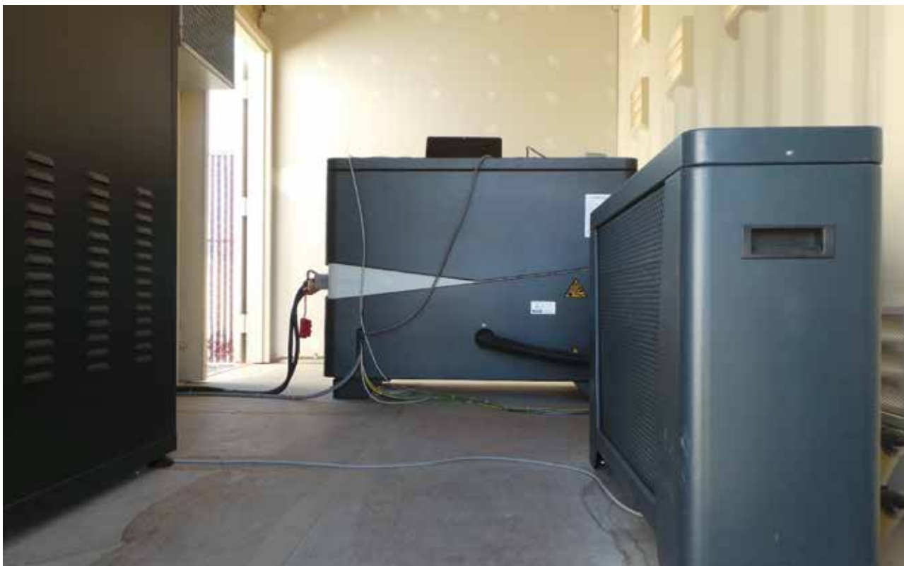
GenCell's G5rx back-up fuel cells installed at a substation for San Diego Gas & Electric (SDG&E). The fuel cell will automatically operate in the event the power grid goes down. The fuel cell can operate 10 times longer than existing back-up power sources, and has the capacity to maintain all substation operations versus only critical operations.
