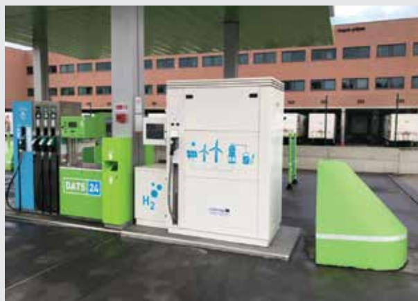
The Colruyt integrated refuelling facility demonstrates the hydrogen refuelling hub model of distributed generation powering facilities, producing hydrogen with the excess power and fuelling both forklifts and trucks and cars at different refuelling points.
