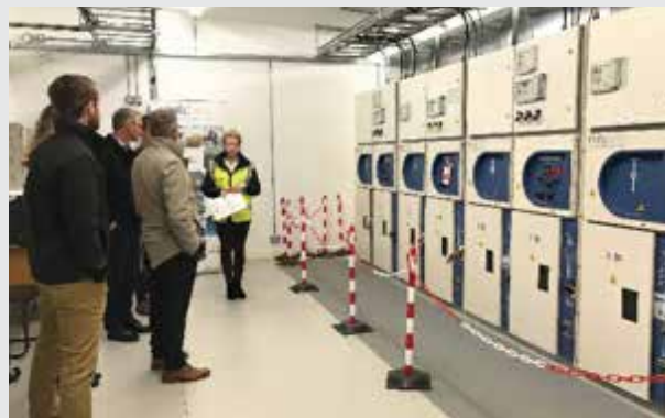
Inside the Billia Croo Site (each machine on the right-hand side is linked to a company wave mechanism off the coast)
