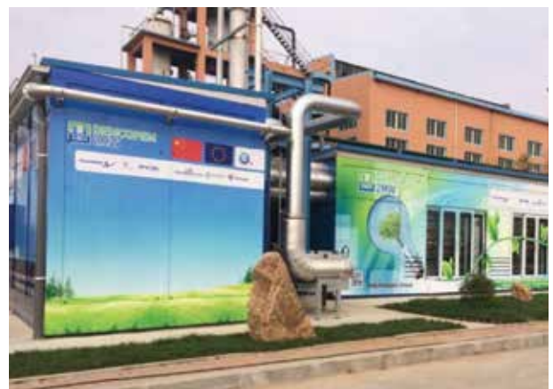
Nedstack has installed a 3.6 MW rated unit capable of delivering 2MW nominal electrical output and up to ~2MW in heat. The unit utilises waste hydrogen from the adjacent chemical process to produce heat and power.
